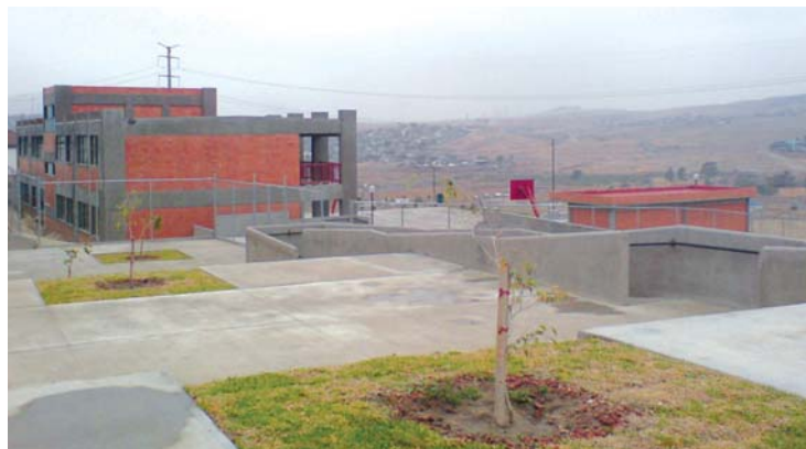
Construction is almost complete on our Mano Amiga school in Tijuana, Mexico.
